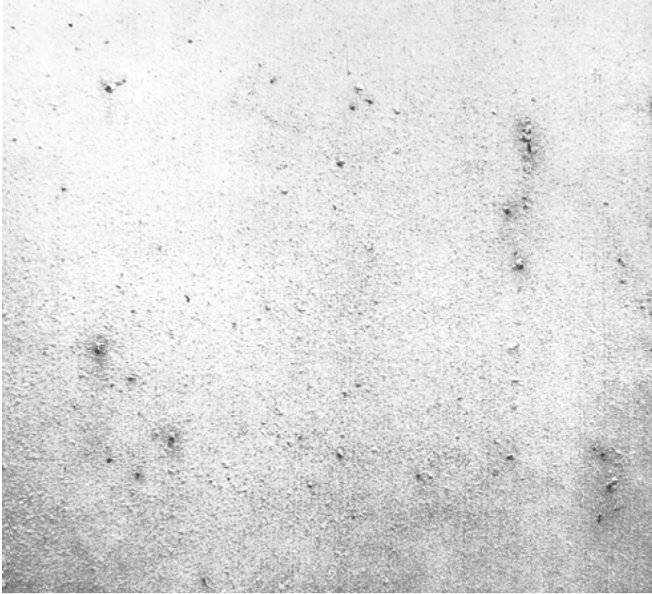
Figure 2 of ISO 4628-3 (Paints and varnishes — Evaluation of degradation of coatings — Designation of quantity and size of defects, and of intensity of uniform changes in appearance — Part 3: Assessment of degree of rusting) Degree of rusting Re1
