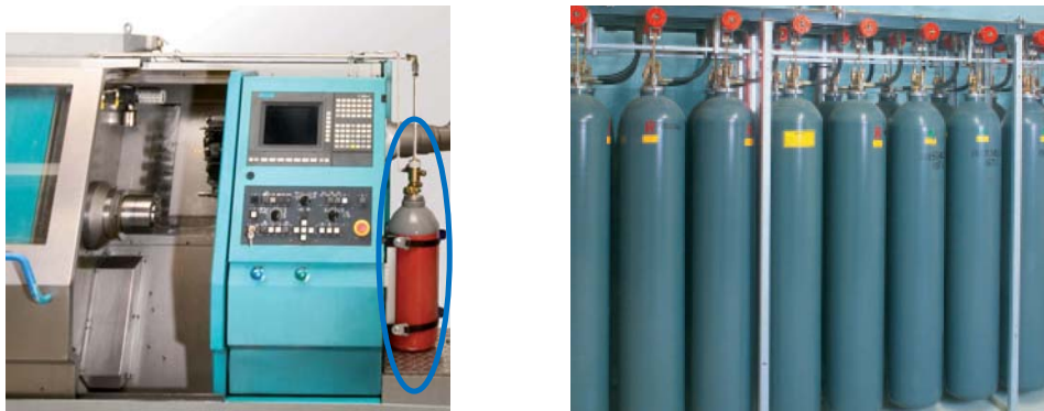
Pictures 4 and 5: Gas cylinders used in stationary fire extinguishing systems
