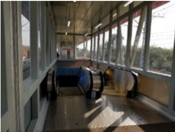
FIGURE 3.28 INSTALLATION OF ESCALATORS AND WAITING HALLS IN RAILWAY STATIONS IN A SIMILAR MANNER TO METRO STATIONS AS PART OF THE EFFORTS AIMED AT THE INTEGRATION OF RAILWAY TRANSPORT INTO THE PUBLIC TRANSPORT SYSTEM OF MOSCOW
