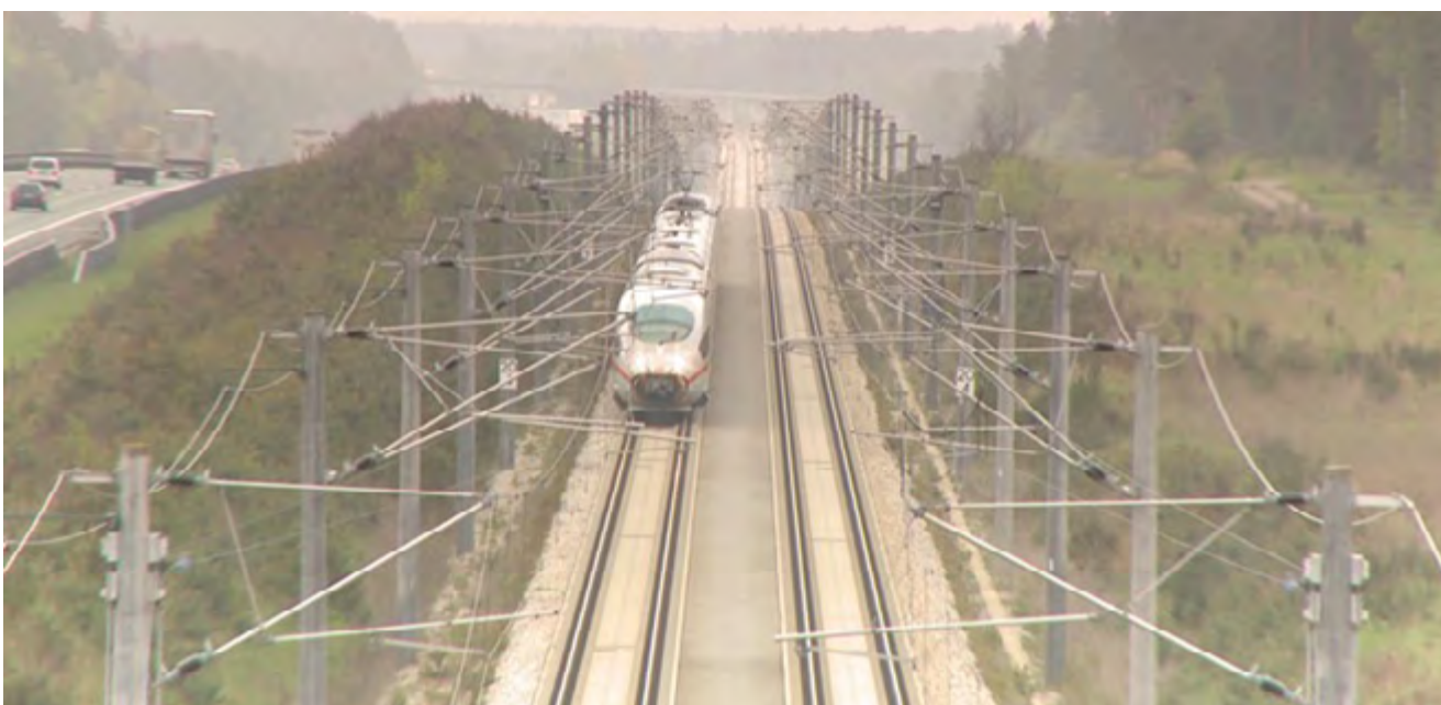
Figure 3.12 - High-speed catenary (ICE)
