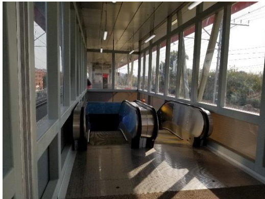
Figure 3.31. Installation of escalators and waiting halls in railway stations in a similar manner to metro stations as part of the efforts aimed at the integration of railway transport into the public transport system of Moscow (Russia)
