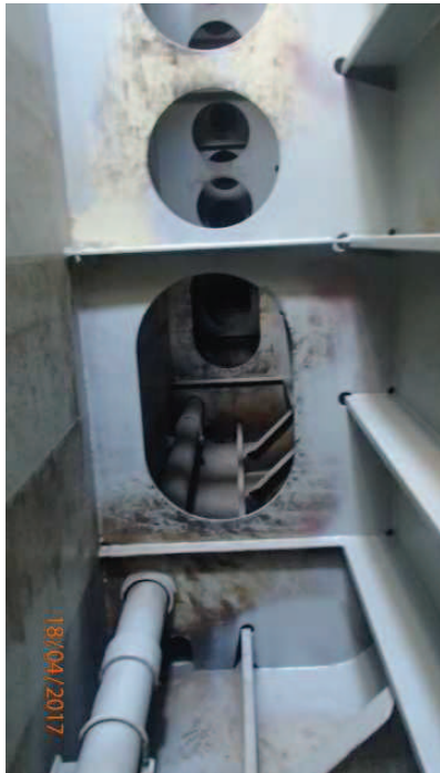
Water Ballast tank no 3, Starboardside (Web frames)
