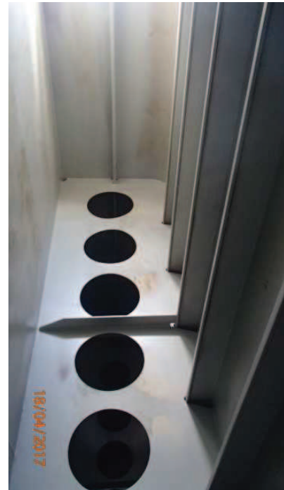
Water Ballast tank no 3, Starboardside (Deck head)
