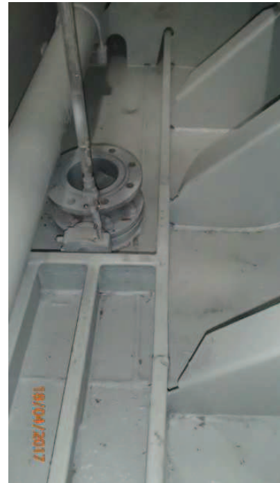
Water Ballast tank no 3, Portside (Bottom valve)
