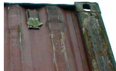
Figure 5.20 Vent tapped over
