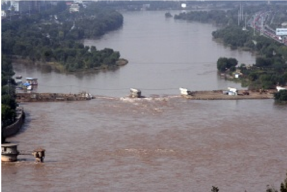
Damaged Harbour Facilities in Lanzhou, Ganxu Province in 2010
