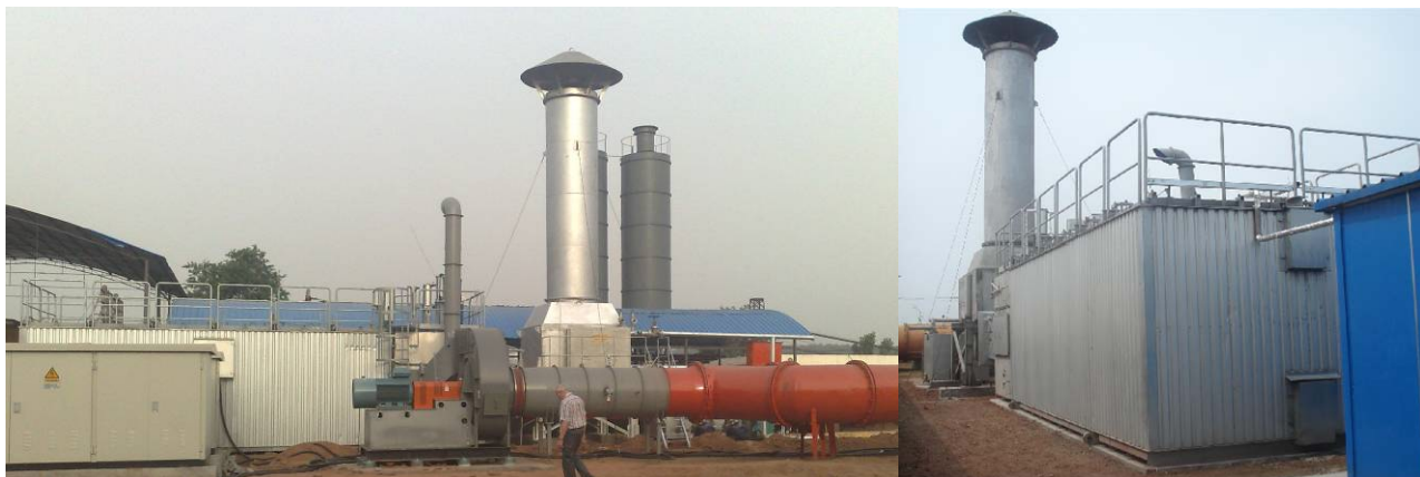
Figure 9.6 VAM Abatement and Energy Recovery Implemented in China
