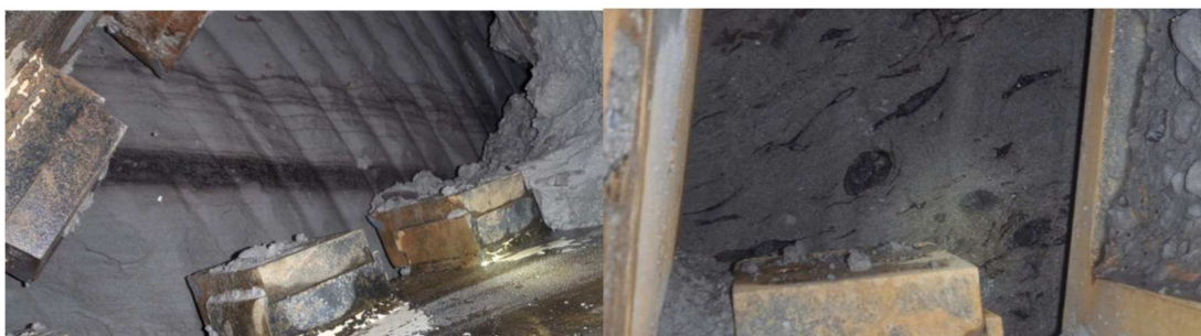
Figure 10: Typical coal lenses (Left) and cutting face (right) of a TBM with specs of coal.
