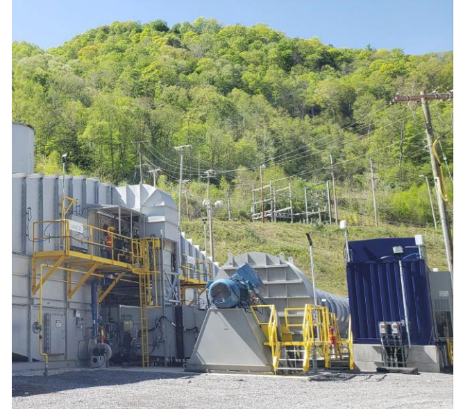
Pump pulling air into the oxidizer
