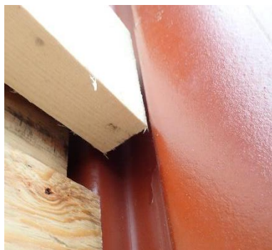
Figure 7.72 Beam too short
