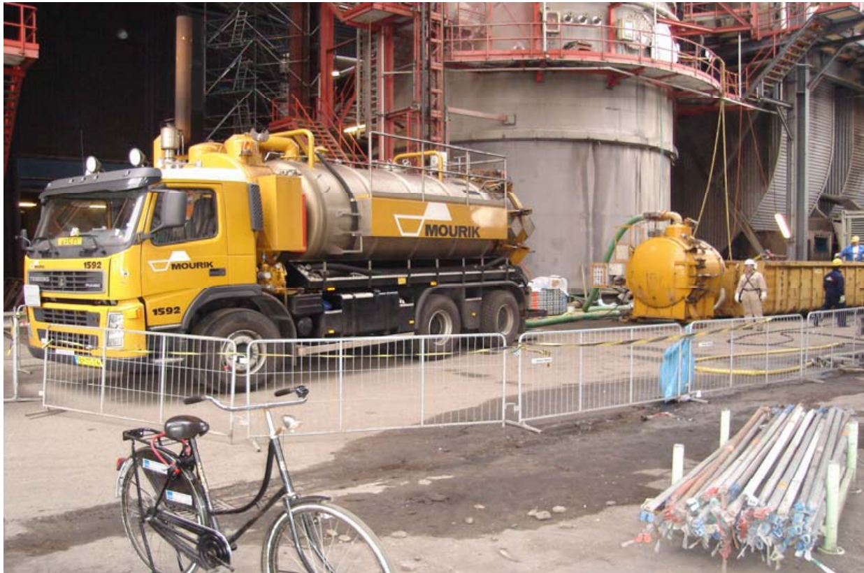
Photo 5: contaminated flue gas desulphurisation plant
