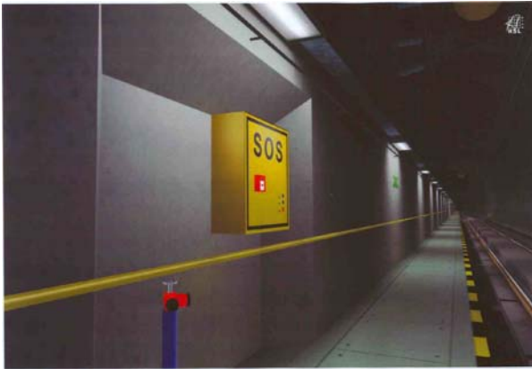
Fig. 10. Connection fire-hoses and S.O.S. facilities
