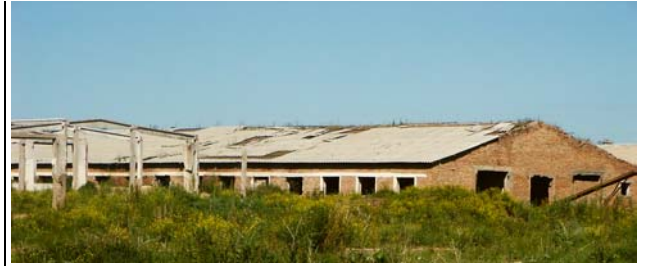
FIGURE 2. Abandoned agricultural buildings suited for large-scale farming are a common sight today (picture taken in Svetlaya Polyana).
