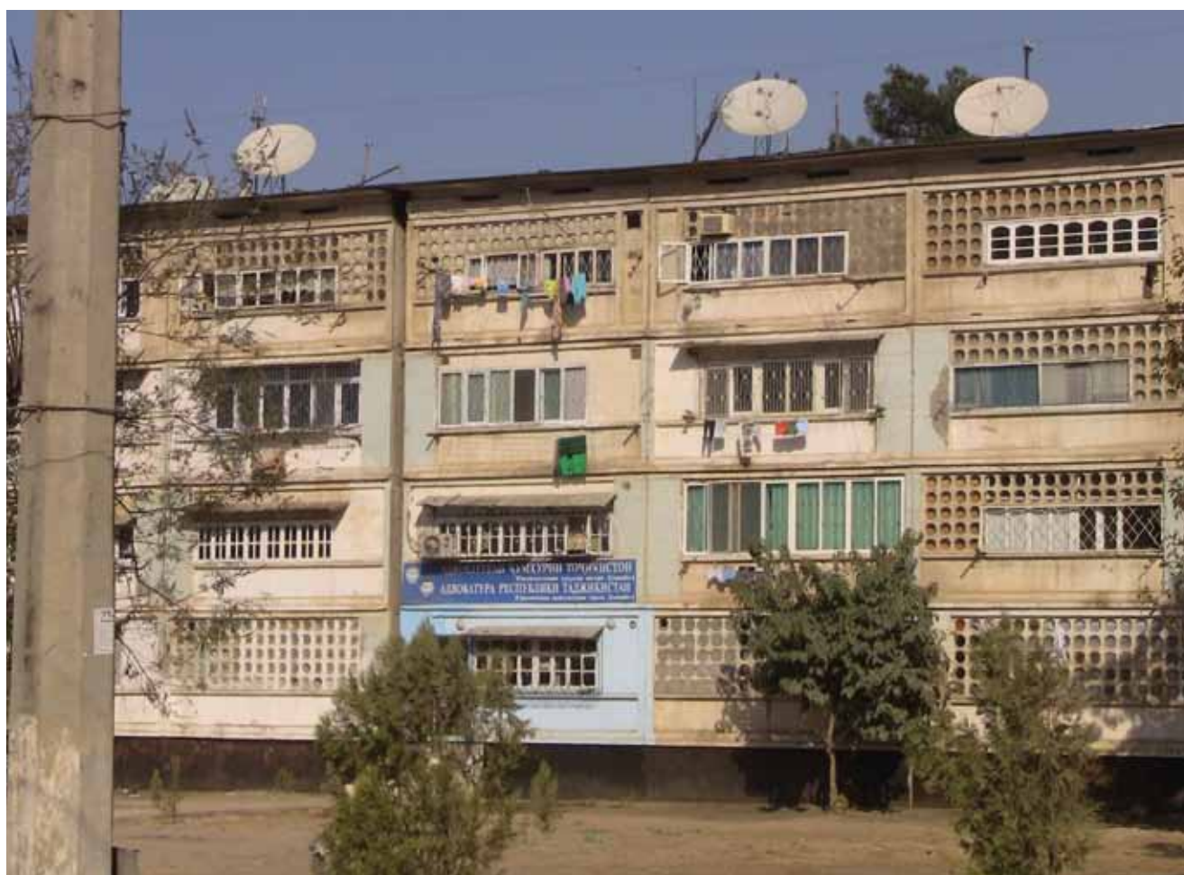
Picture 3. Multifamily housing in need of upgrading
