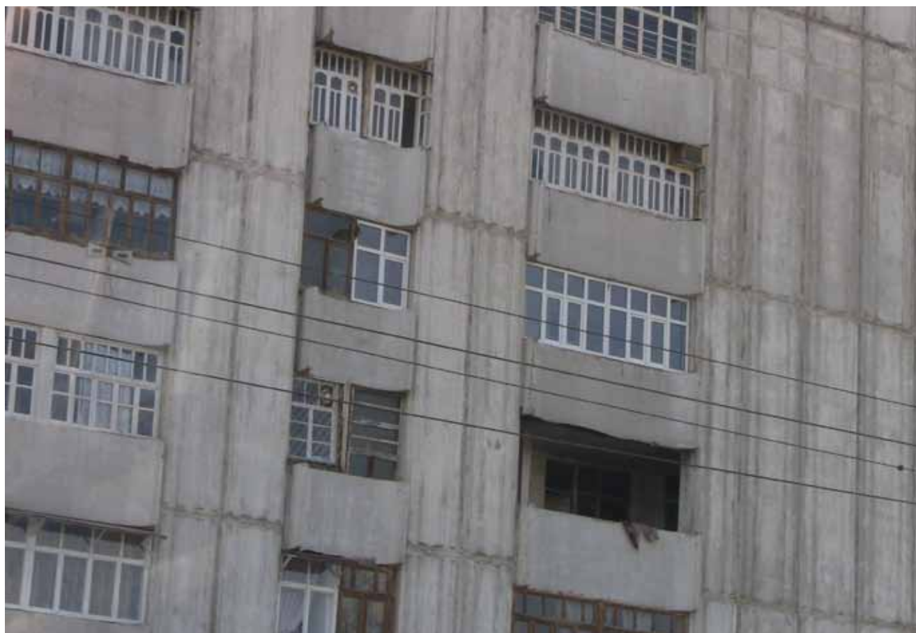
Picture 4. Multifamily housing in need of upgrading
