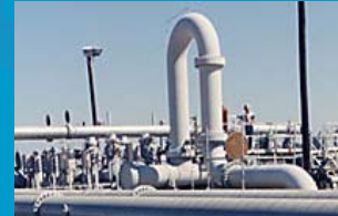
Natural Gas Pipeline/ Town Gas
