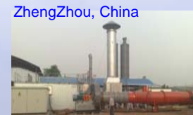
Abatement/hot water ZhengZhou, China
