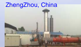
Abatement/hot water ZhengZhou, China
