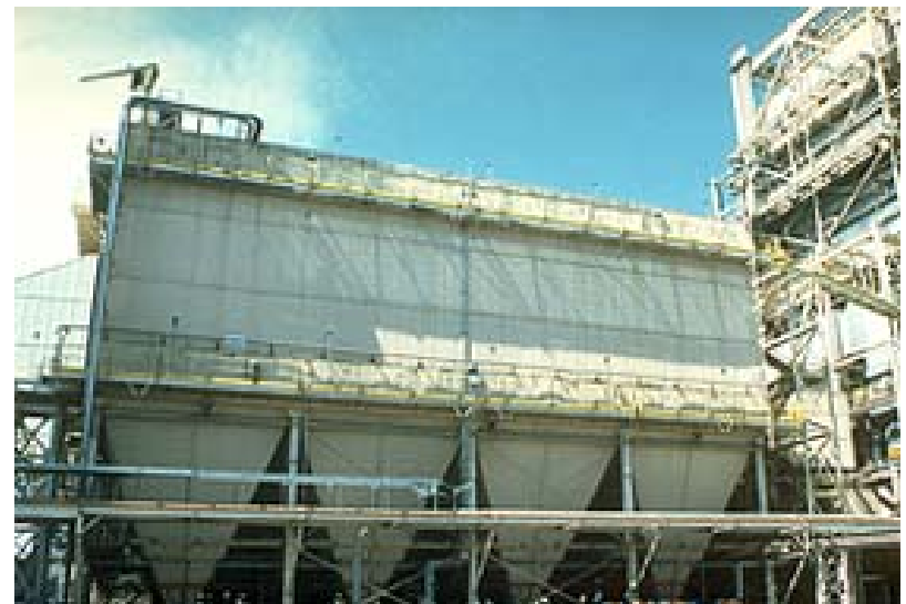
Nevada Power Company Reid Gardner Unit 4 - 245 MW Moapa, Nevada, USA
