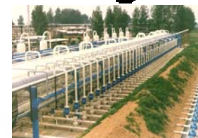
MOL Natural Gas Transmission Plc.
