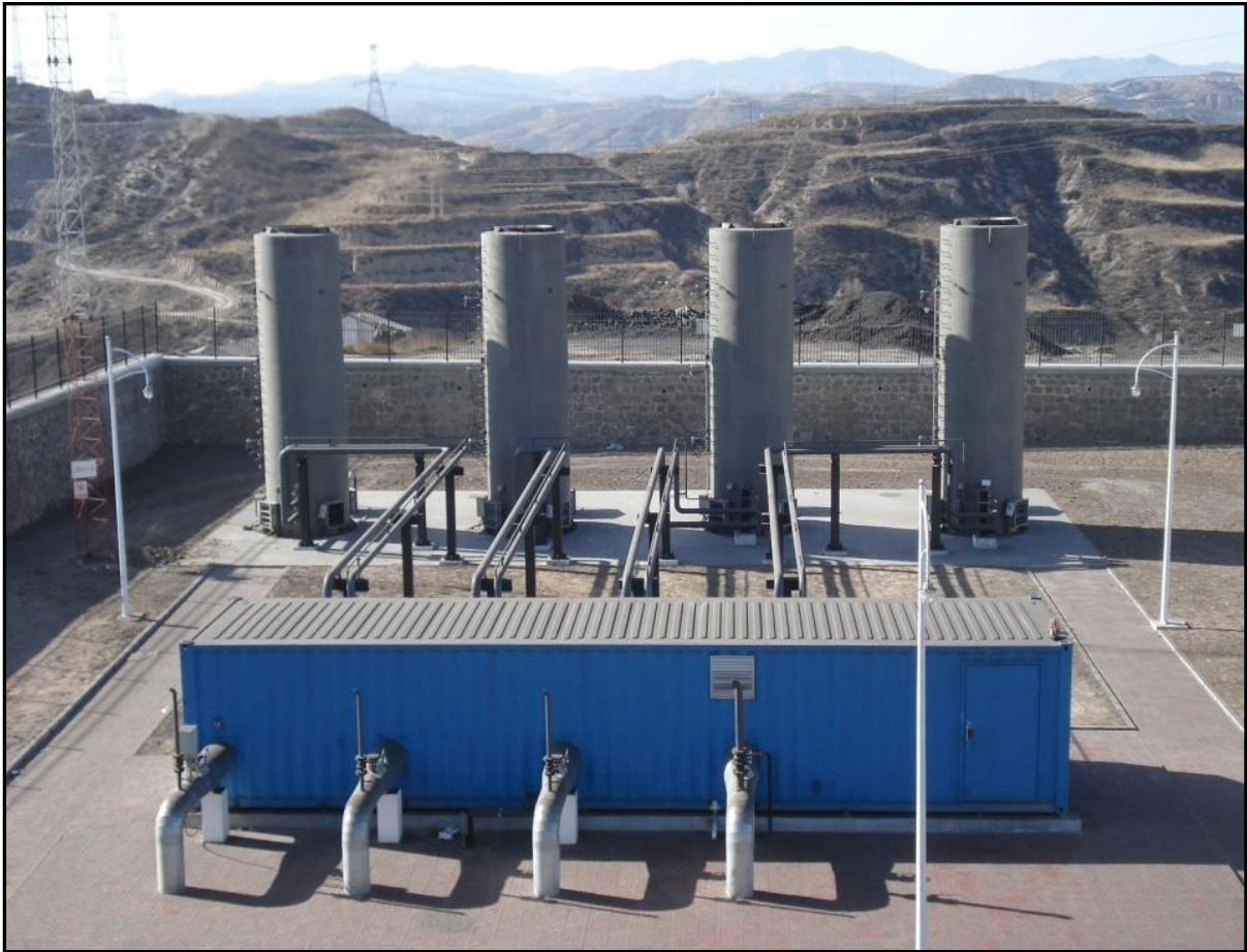
Figure 2. Flare system at mine T
