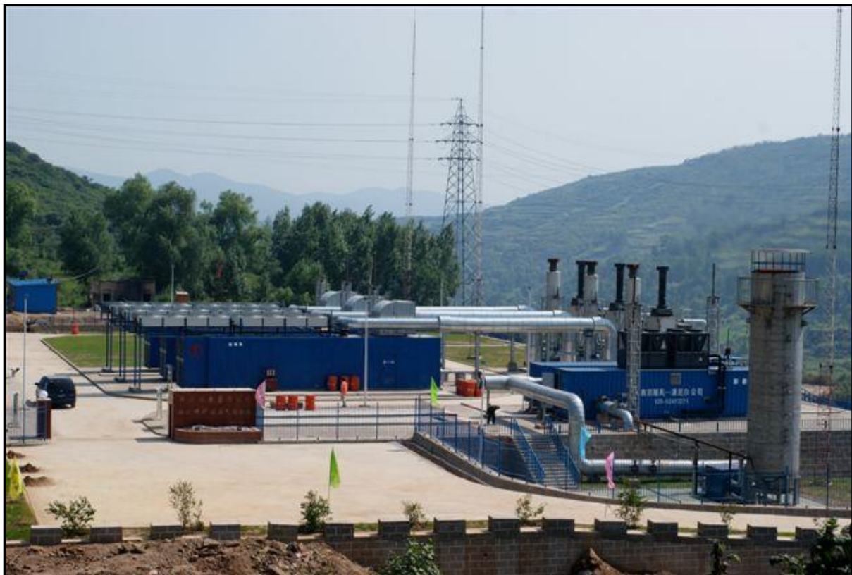
Figure 1. CMM co-generation power plant phase 1 at mine D
