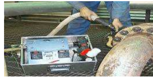
Oil and Gas Systems
