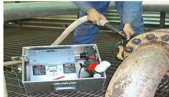
Oil and Gas Systems
