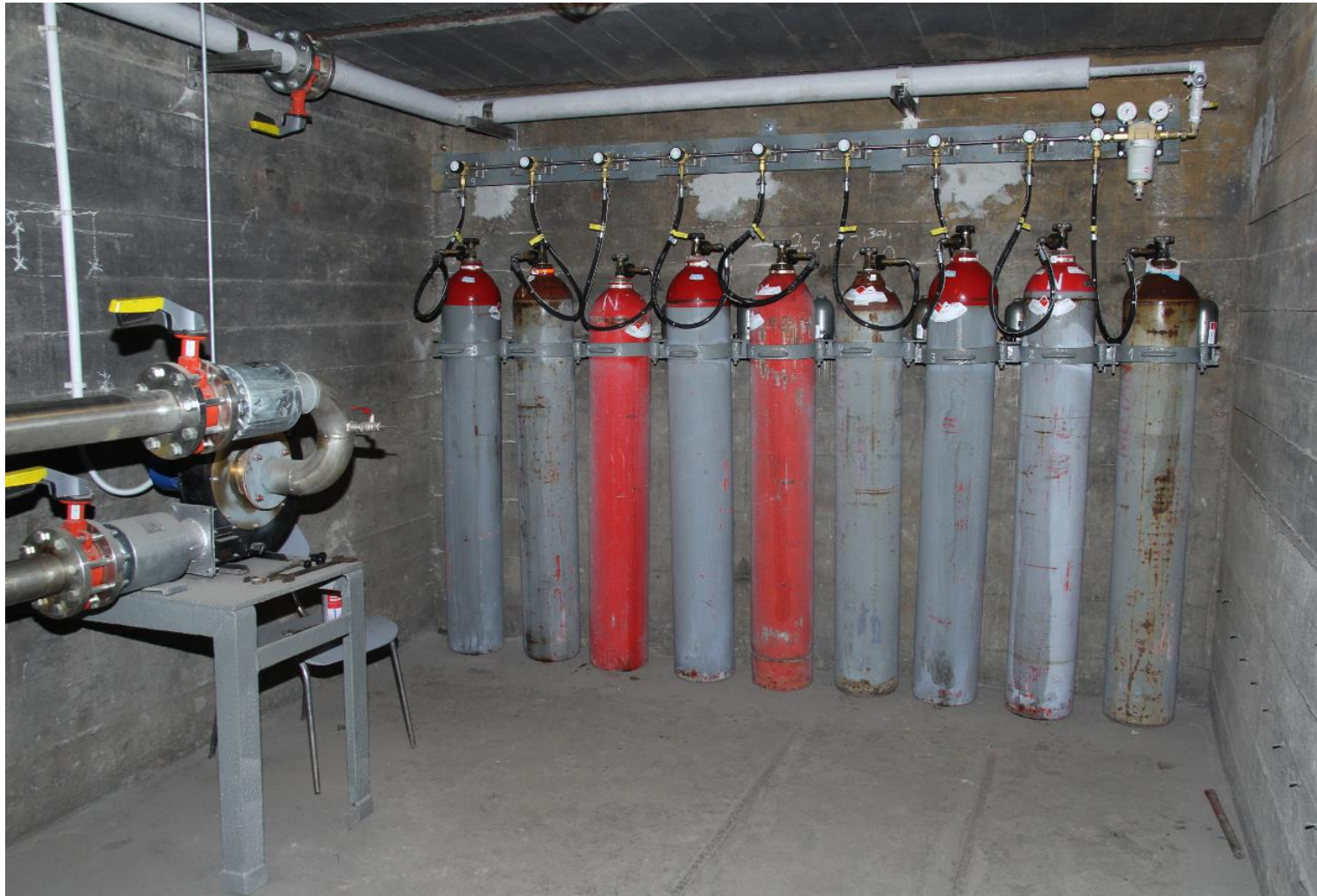
Underground methane supply chamber
