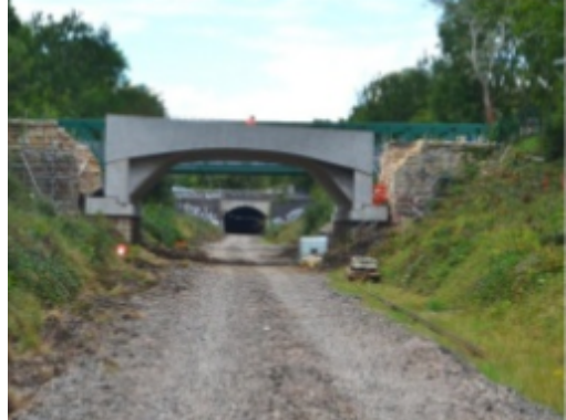
Slide from "Oxford Club of Constructing Excellence" Graham Cross, Chiltern Railways 14 January 2016
