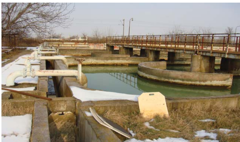
OHIS wastewater treatment plant
