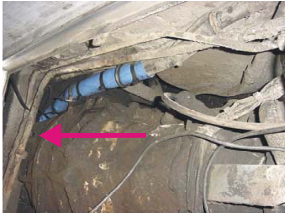
Figure 2. Protection and tightening of the battery cable at the repair shop. The wiring loom has been protected from abrasion with protective tubing and supported well. (Photo : Oy Pohjolan Liikenne Ab)
