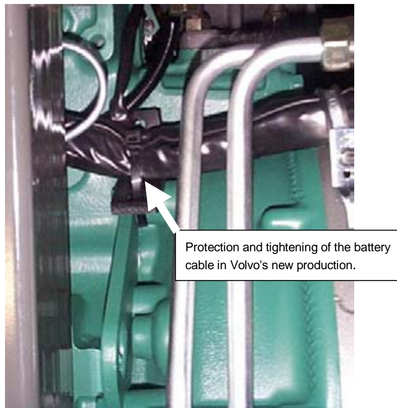
Figure 3. The tightening of the cable in Volvo's new production. The hoist bracket is below the tightened cable. (Photo : Volvo Ab)
