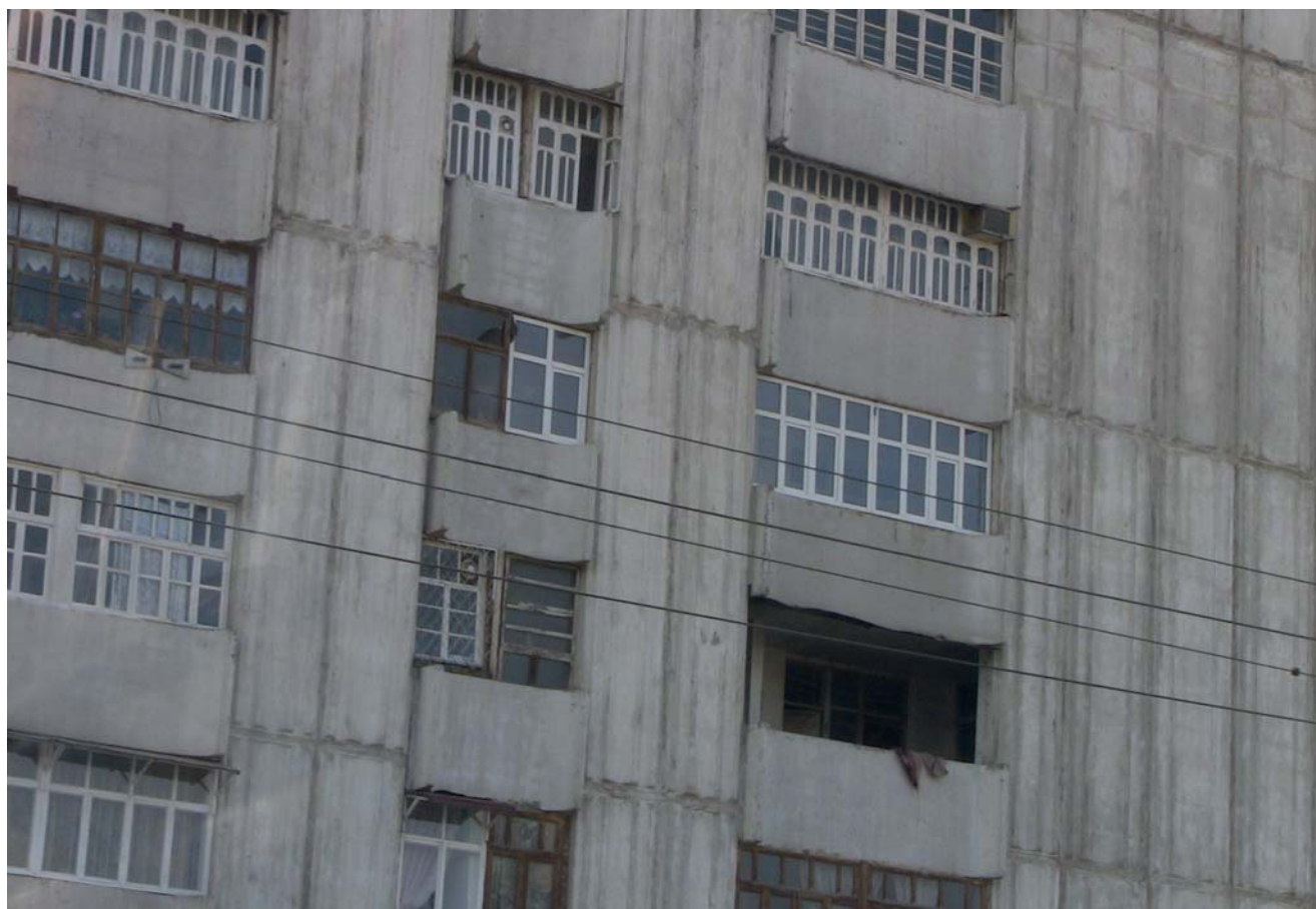
Picture 4. Multifamily housing in need of upgrading
