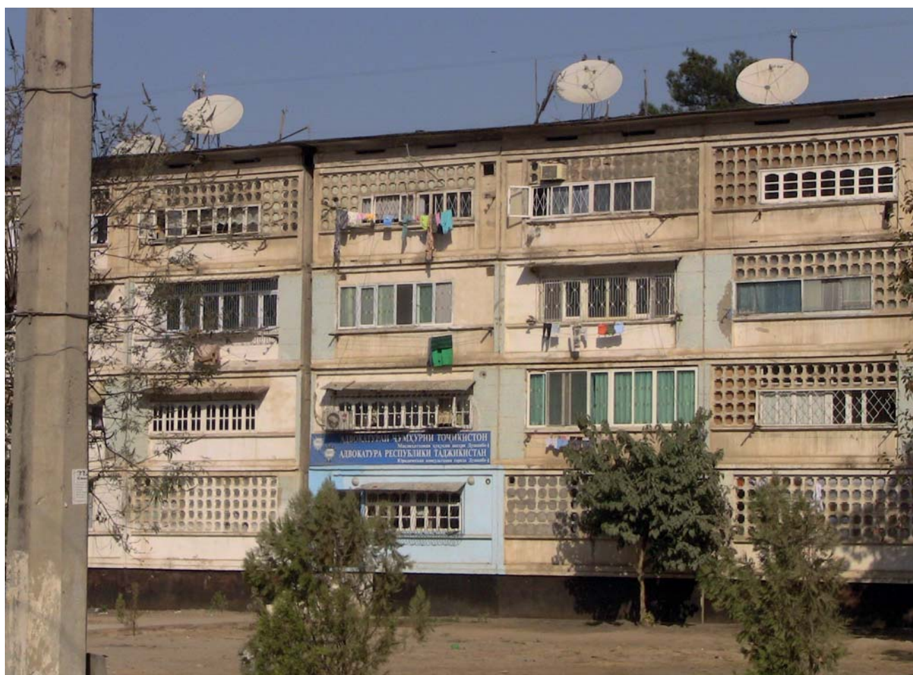
Picture 3. Multifamily housing in need of upgrading
