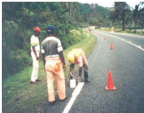
Plate 1 (left): Road marking to improve safety.
